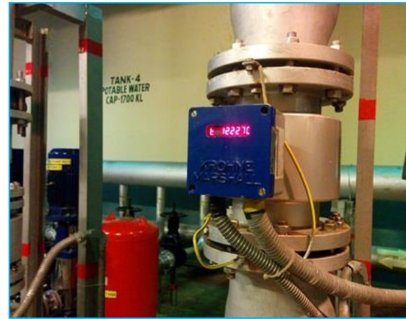
System level Water Metering facility
