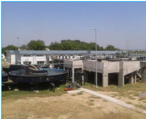
16.6 MLD Sewage treatment plant
